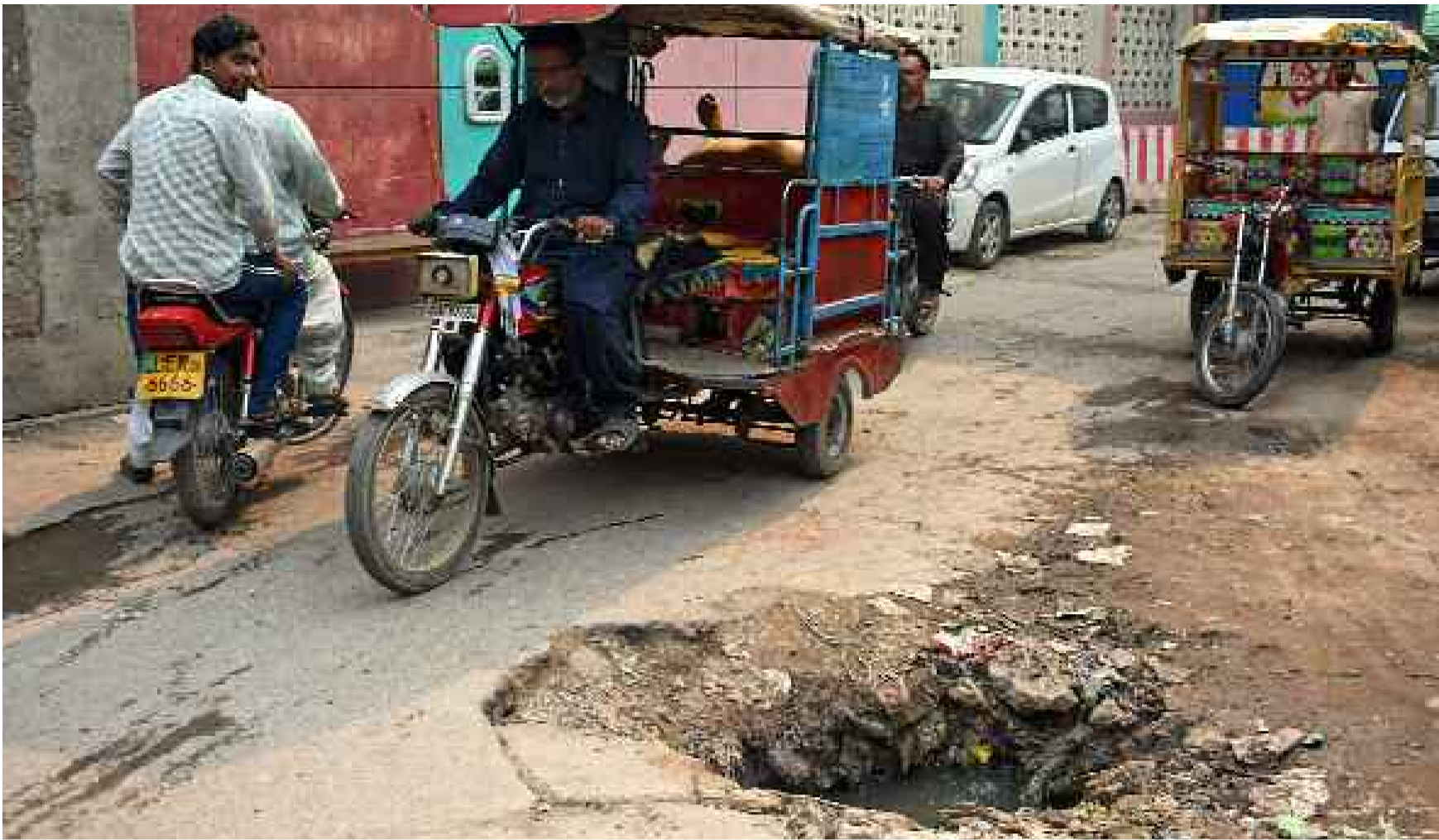
LAHORE: People facing difficulties due to open manhole at tyre market. —Online
