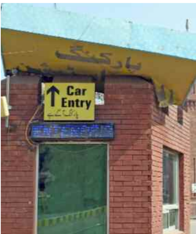
LAHORE: A view of broken parking sign board fell down on a CCTV camera outside Lahore Railway Station.
