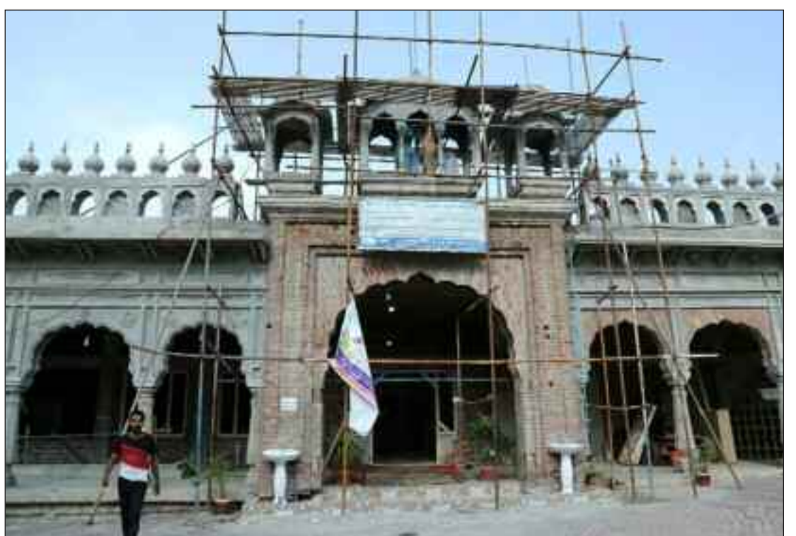
LAHORE: Renovation work underway at Gurdwara Dera Sahib. It is a Gurudwara which commemorates the spot where the 5th Guru of Sikhism, Guru Arjan Dev was martyred.
