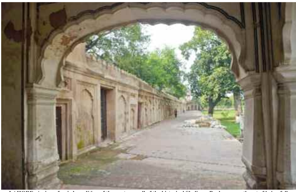
LAHORE: A view of weird condition of the western wall of the historical Shalimar Bagh, poses a threat of being fallen any time, which needs attention of the concerned authorities. —Online
