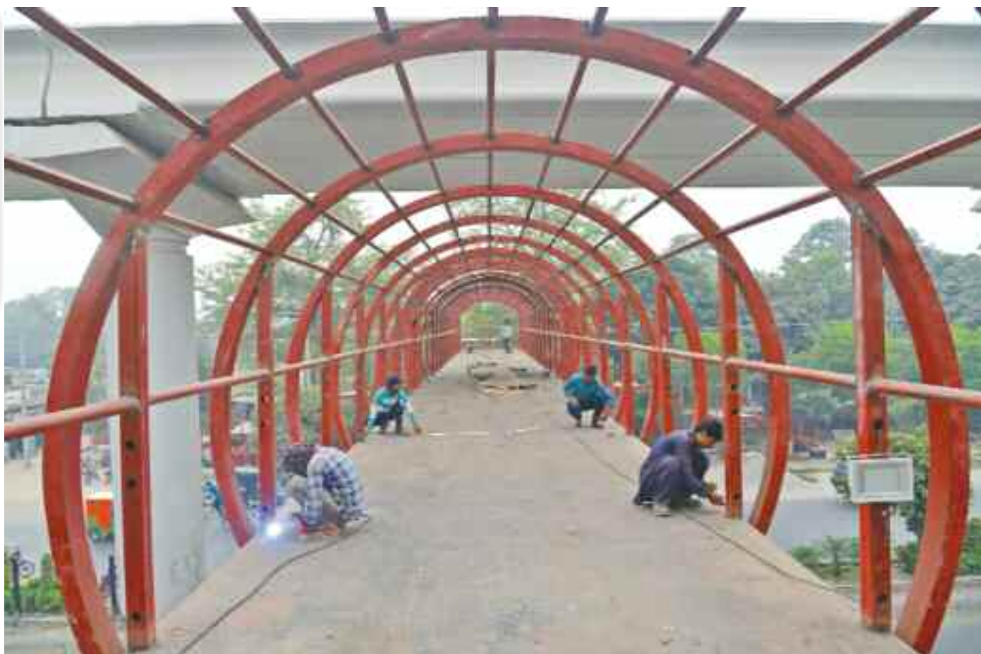
LAHORE: Labourers busy in their work at the newly constructed overhead pedestrian bridge for the students of (UET).
