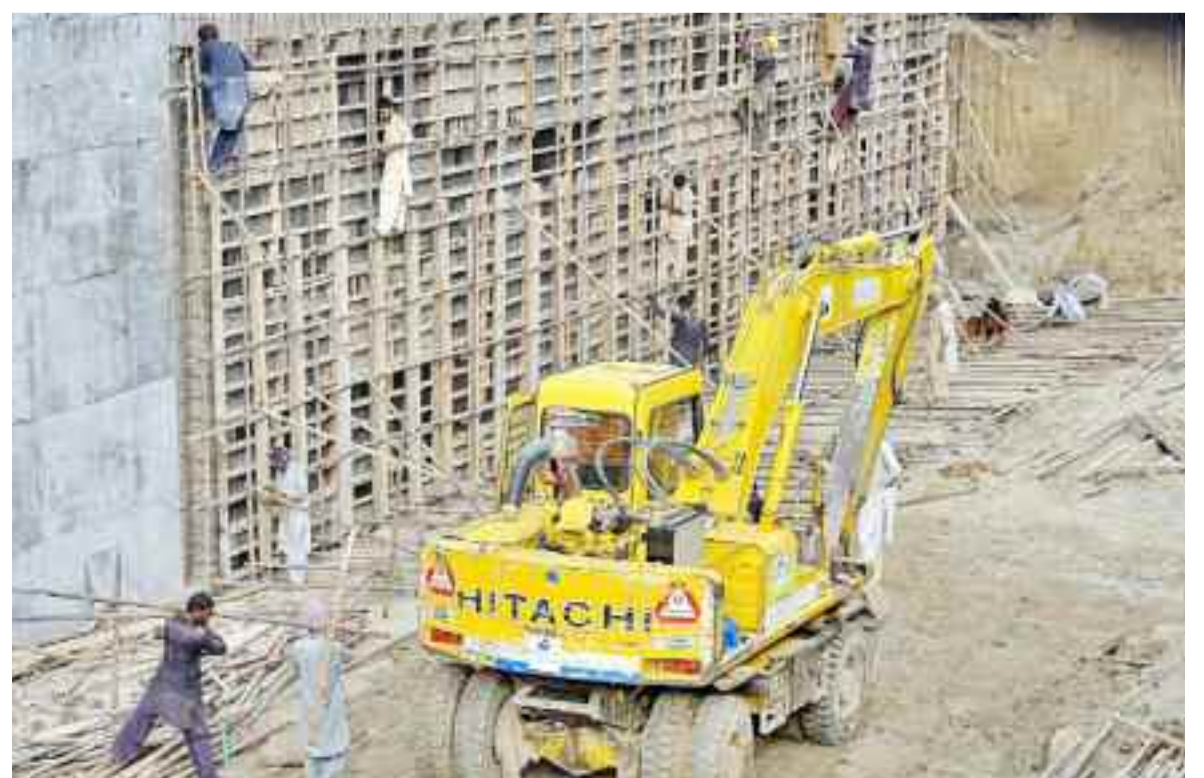
LAHORE: A view of construction work of Firdous Market Underpass during development.
