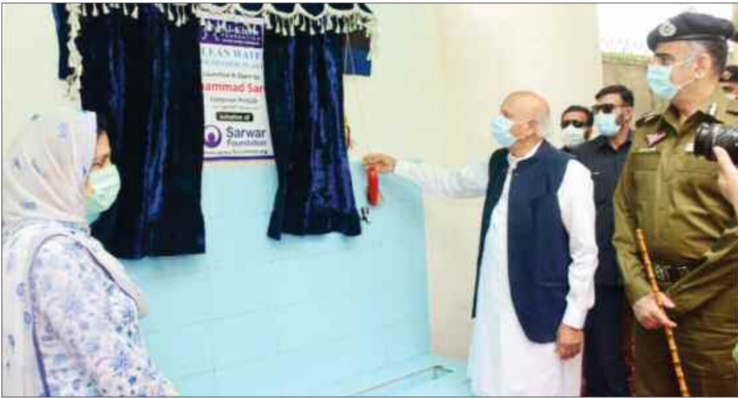
LAHORE: Punjab Governor Ch Muhammad Sarwar inaugurates water filtration plants intalled by Sarwar Foundation and Al-Khair Foundation at the Central Police Office.
