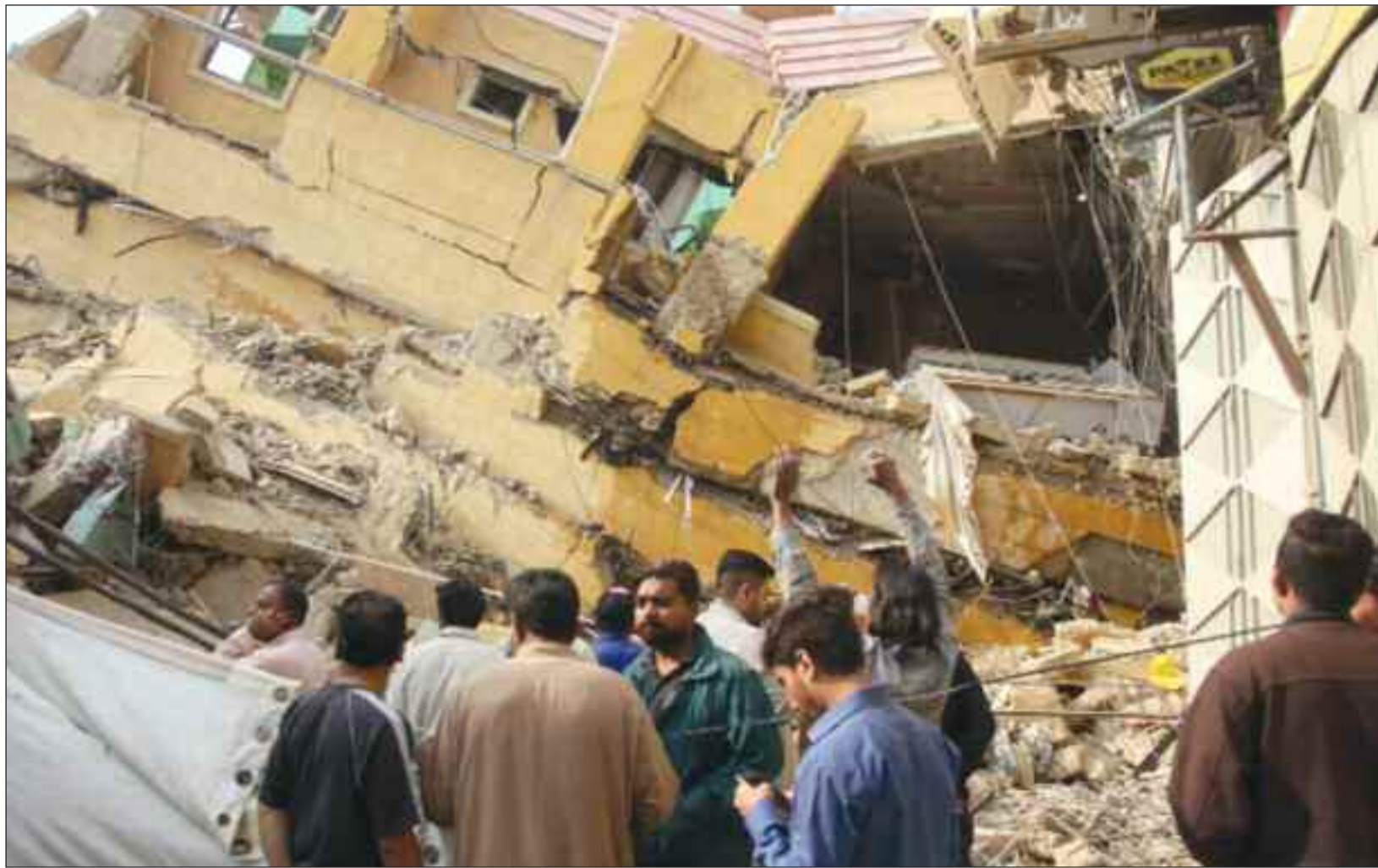
KARACHI: A view of building collapsed in Karachi's Timber Market in afternoon hours. It was constructed 15 years ago. The Sindh Building Control Authority had gotten the six-storey building the vacated. It comprised 21 apartments.
