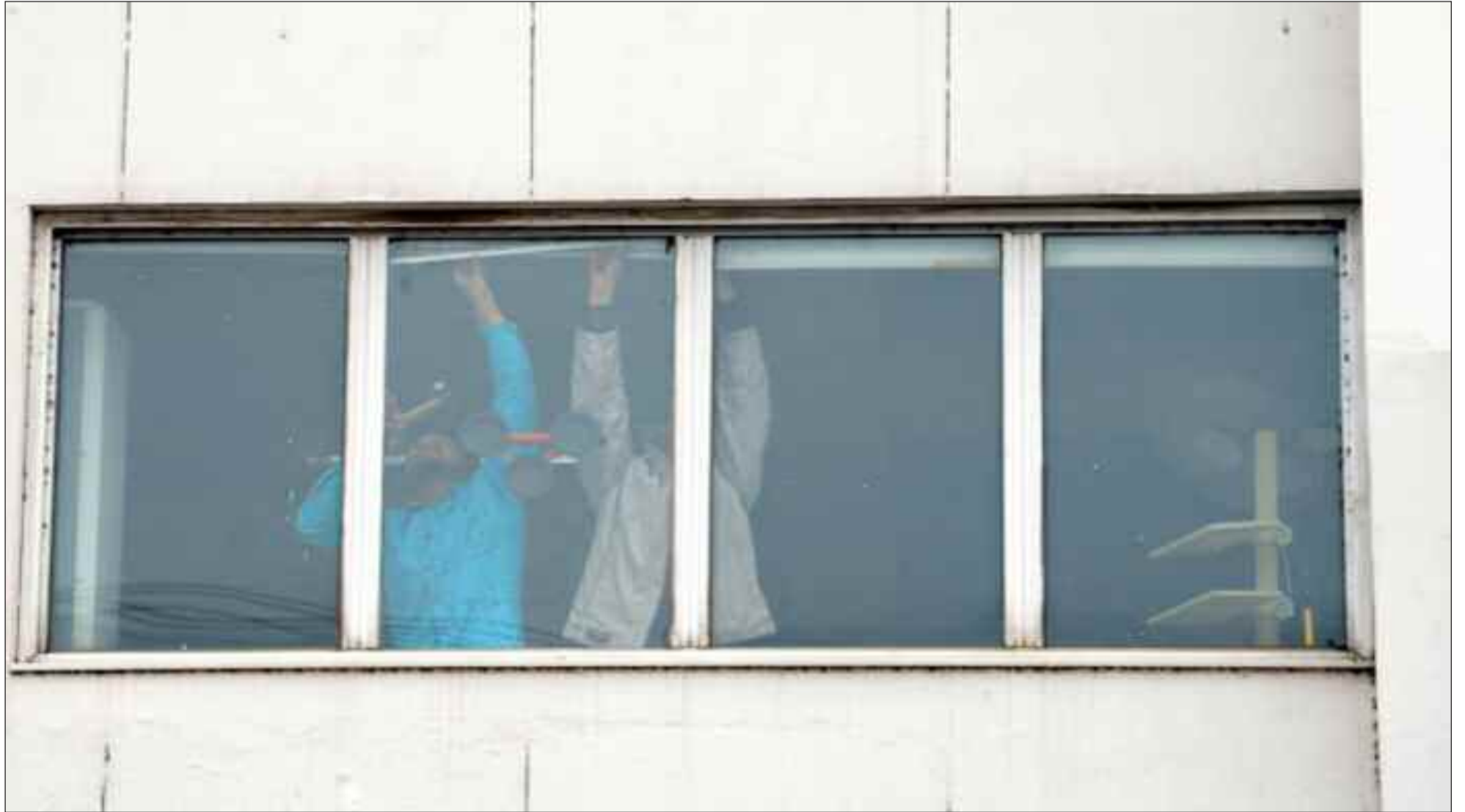
LAHORE: Workers busy in repairing of windows mirrors of the Punjab Institute of Cardiology (PIC) as after the attack of lawyers on hospital. —Online
